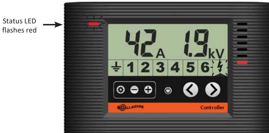
Controller showing the energizer in current alarm
